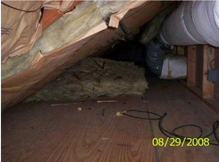
Insulation batts have fallen out of position-properly reinstall
