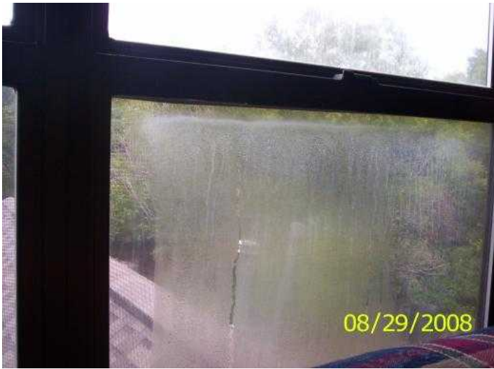
Moisture present inside the layers of glass, south window
