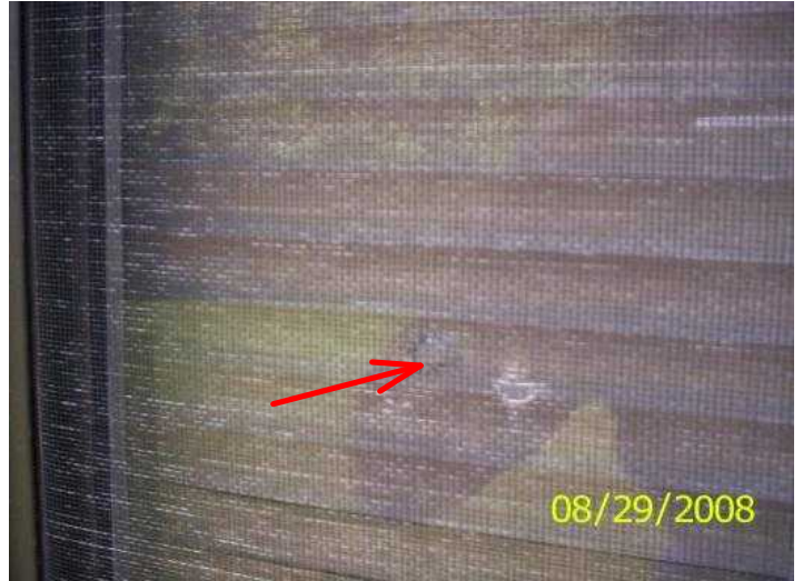
Cracked, broken or missing glass ,north bottom window by garage door .
