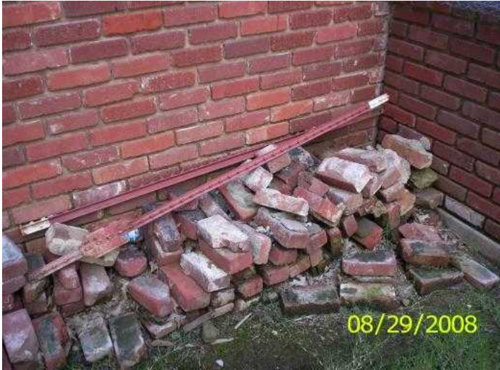
Bricks and mortar piled against wall , possible safety hazard and possible insect
