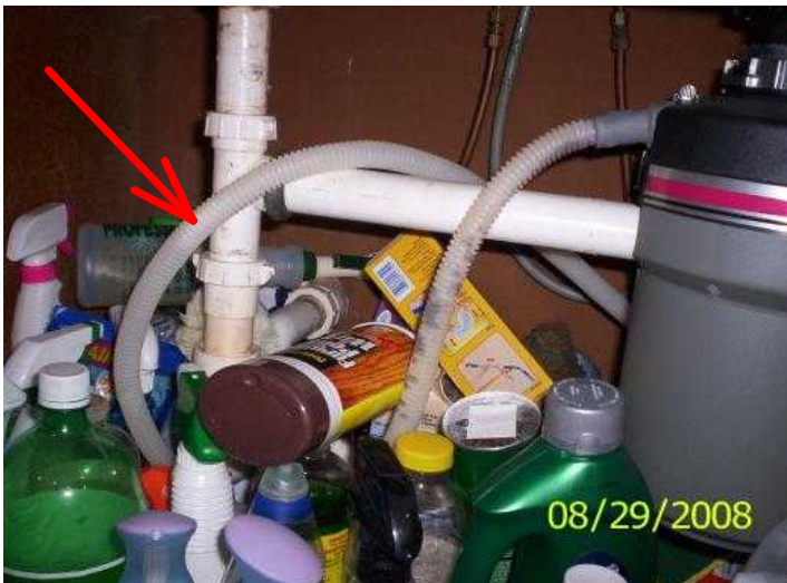
Air gap hose improperly connected
