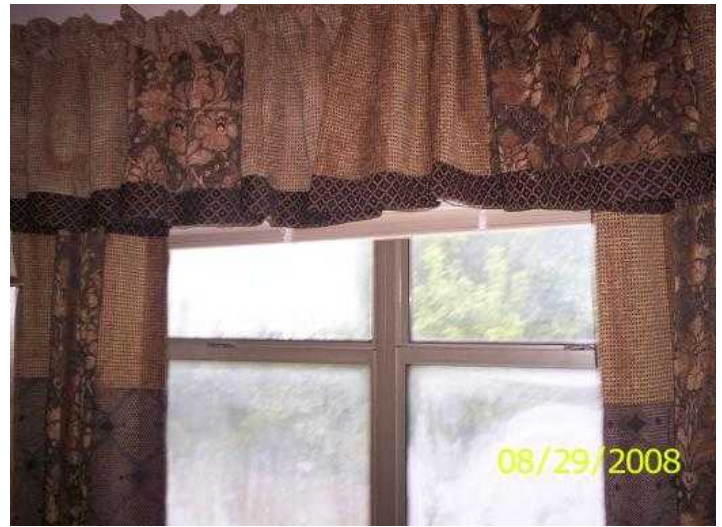
Both west windows will not open. Window has fogging between the layers of glass, all windows in the sitting area.
