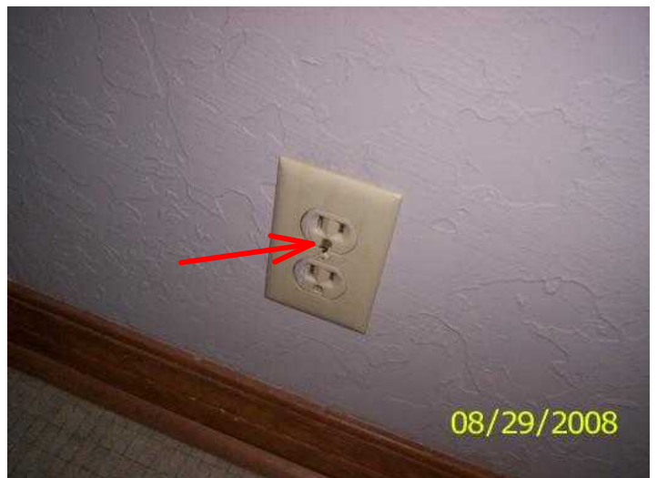
Non-GFCI circuit by sink. Plug by toilet has ground broken off in it.
